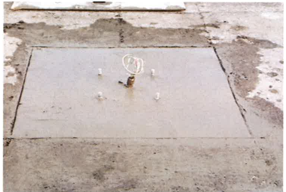
Inground Pad with Electrical Only
