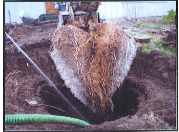
This photo shows root intrusion in a septic tank.
